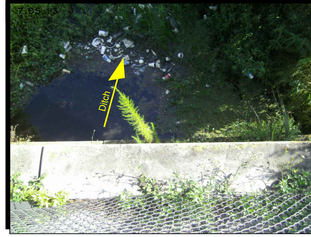
Photo 6) View Looking Downward from Atop of Outfall - West Lakeland Business Park Phase 2
